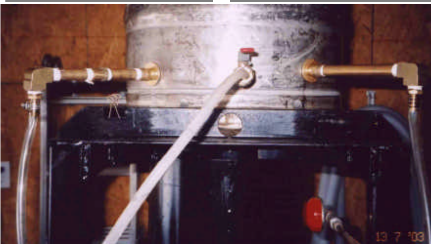
Hot Liquor Tank (Exterior View)
